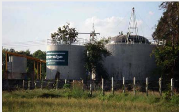
Große Biogasanlage in Ubonthani, Thailand
